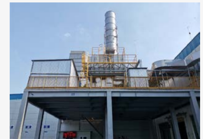
Coating Waste Gas Emission Reduction Facilities
